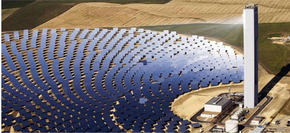
Concentrating Solar Plant, California
